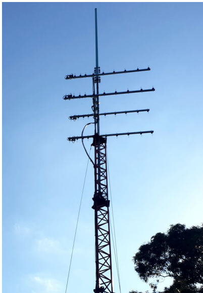
4 x 11el 477MHz LFA Yagi installed at one of our Oz customers
