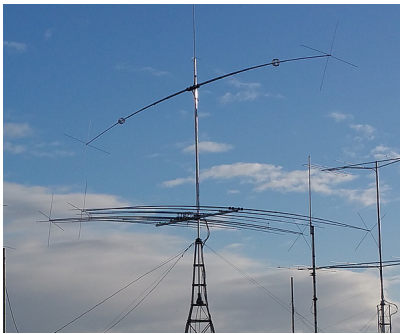
The Delta C-140 installed above an XR6 on top of Europe's Ham Store - Waters & Stanton
