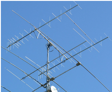
A pair of 20el LFA Ultra Xpols installed at OE5KE
