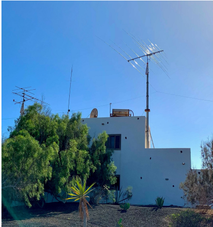
The XR7 installed at EA8BFK
