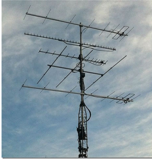
2 x 8el 144MHz LFA installed at G1MHU
