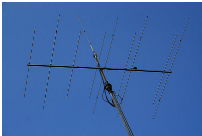
The 9el Duo installed at MOSAT
