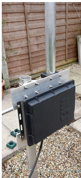
A typical installation with MFJ tuner installed (VertiGo 43V pictured). Optional ATU mount fitted
