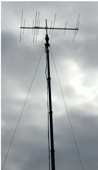
The 12el Duo installed at M0VOZ
