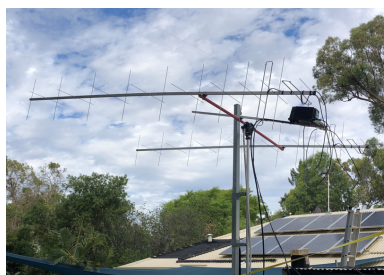
A pair installed at VK6JX
