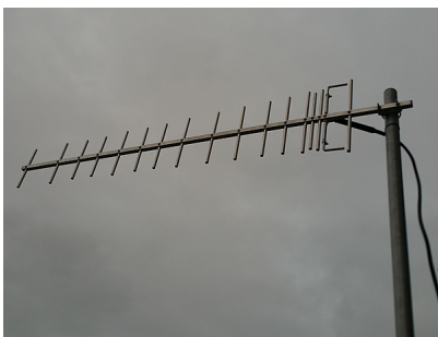
1 x 17el PMR 446 Yagi installed
