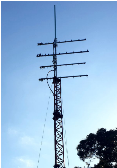
4 x 11el 477MHz LFA Yagi installed at one of our Oz customers
